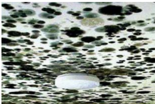
Black mold can be a homeowner's worst nightmare.
